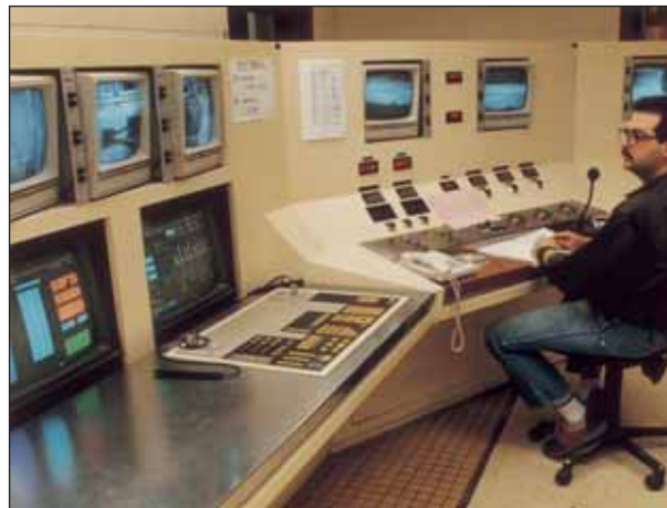
A control room, such as the one seen here, can be found in a modern float glass manufacturing facility. Here, the forming glass can be monitored throughout the entire process.
