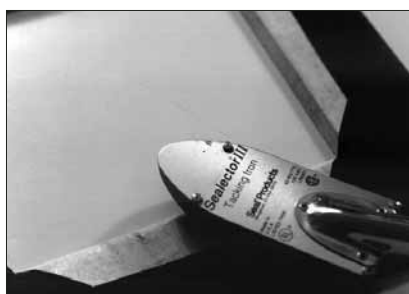
Photo 8: Mount the bark paper to the face of the created 8-ply blunt cut window opening, remove center, miter corners, and wrap to the back of the opening with a tacking iron.
