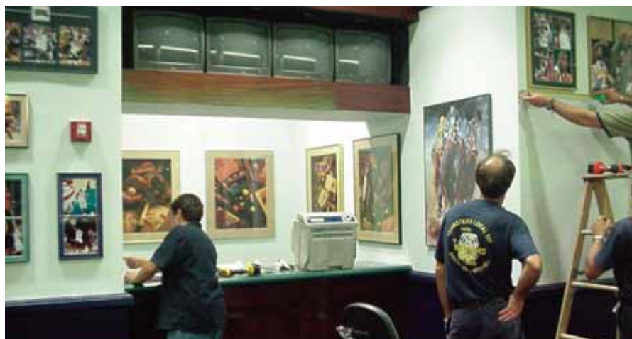
Photo 3: Sports memorabilia was also installed onto the walls in the room with hinged iron gates.
